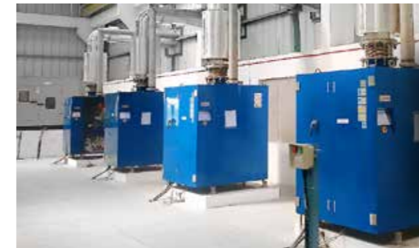
Anjar Wastewater Treatment Plant (India) Optimisation: supply of the activation Technology: Aerzen Turbo 4 x AT200 0.85 Wastewater: 30.000 m 3 /day Size: ? Savings: 25% energy/35% space saving
