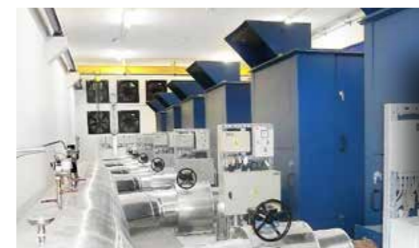
Industrial Wastewater Treatment Plant Sloftnaft refinery (Poland) Optimisation: purification stages Technology: Delta Blower 6 x GM90S Wastewater: 35.000 m 3 /day Invest. volume: €1.3 million Savings: €280,000 annually
