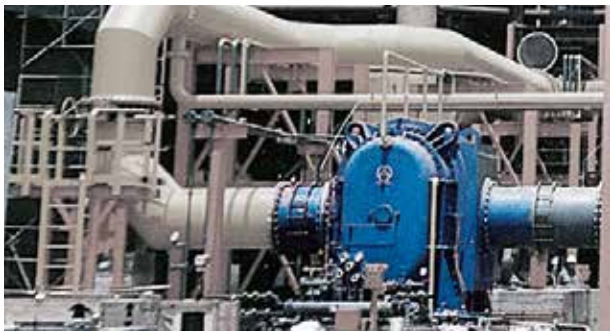
Plant for pneumatic conveying of bulk materials
