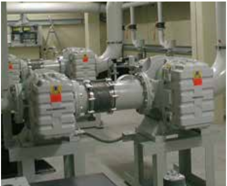
3-stage pumping set for 2 x 12,000 m³/h in vacuum coating technology
