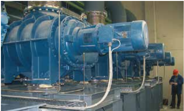
4-stage vacuum plant with 2 x 30,000 m³/h intake volume flow in steel degassing
